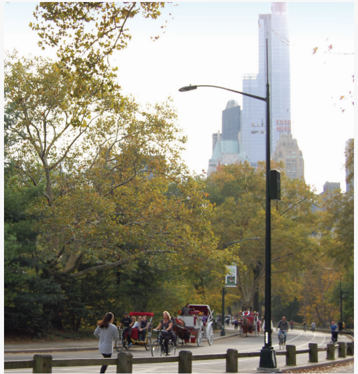
Small cell installation on a Central Park streetlight.
